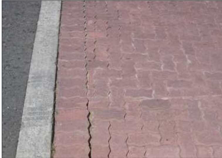
Figure D.3: Pumping adjacent to edge restraint as a result of poor drainage
