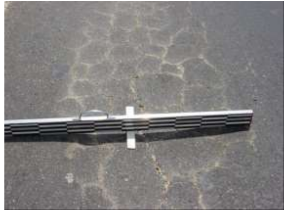
Figure A.8 Rutting originating from the upper pavement layers
