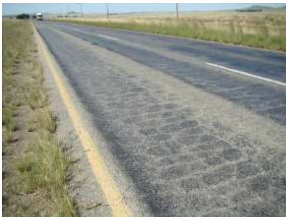
Figure A.7 Rutting originating from thick asphalt surface layer
