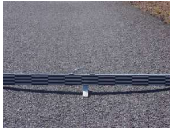
Figure A.9 Rutting originating from the lower pavement layers
