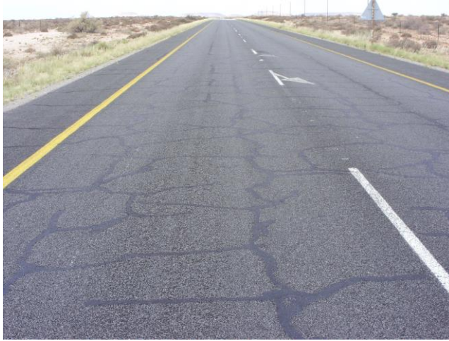
Figure 14: Typical pattern of stabilization cracking
