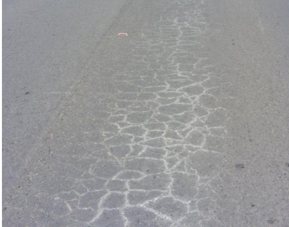
Figure 18: Typical crocodile cracking and pumping associated with overstressing of a stabilized base
