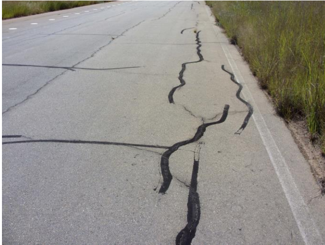
Figure 16: Reflection cracking of stabilized subbase through 150 mm G1 base and 25 mm asphalt
