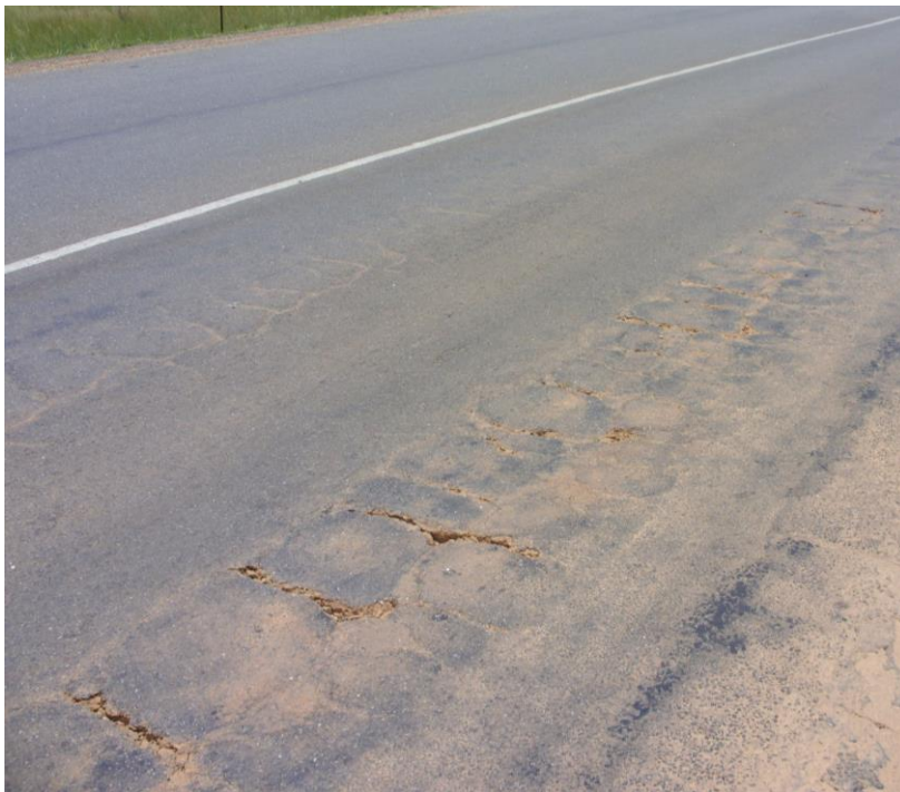
Figure 17: Typical cracking due to overstressing
