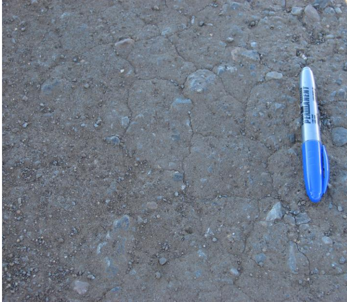
Figure 20: Cracking of an old stabilized layer seen during rehabilitation (equivalent granular phase)
