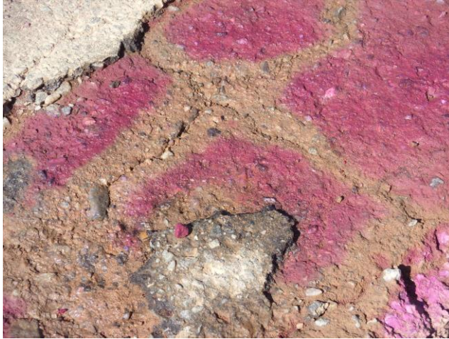
Figure 25: Carbonation along cracks in top of the base
