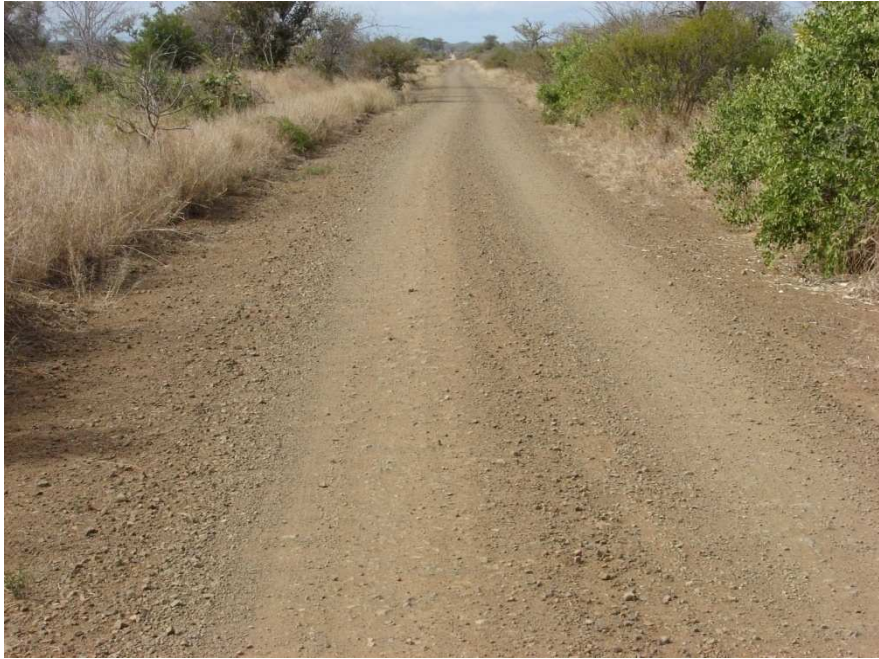
Figure 2 Loose stones on wearing course surface
